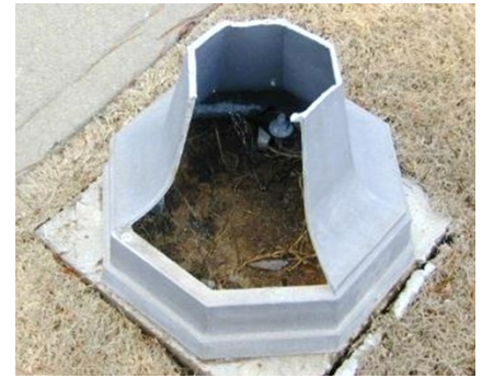
3.) Radarsign's pole base broke away from the sign pole on impact as it was designed to do.
